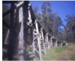
h01439 rail bridge over monbulk creek selby towards menzies creek she project she
