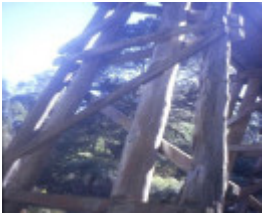
h01439 rail bridge over monbulk creek selby supporting beam she project she
