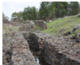
Partial collapse of Bessiebelle July 2013
