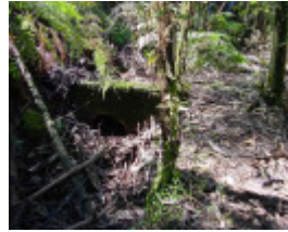
Mt Evelyn Water Supply Pipe
