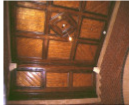
former albert park railway station complex ferrars street albert park ceiling detail jun1998
