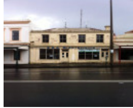
Appearance prior to repairs in 2013
