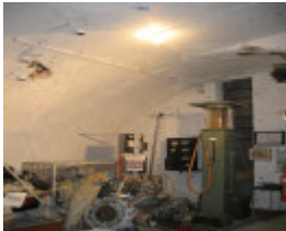
Internal view of engine room, Feb 2008.
