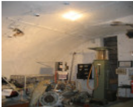
Internal view of engine room, Feb 2008.
