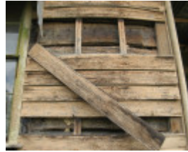
Castlemaine military quarters_slabs under weatherboards_KJ_7 Feb 08
