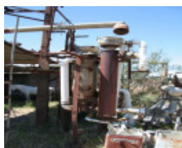
Condensers Eucalyptus Factory Inglewood Oct 2006
