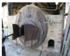
Boiler Eucalyptus Factory Inglewood Oct 2006
