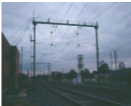
h02025 6 bunyip sub stationjul03 jc
