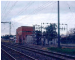
h02025 3 bunyip sub stationjul03 jc
