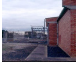
h02025 2 bunyip sub stationjul03 jc
