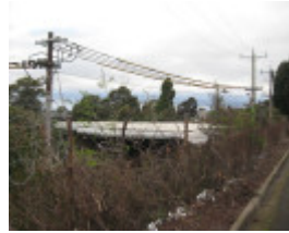
Maribyrnong substation view from above
