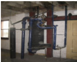
61-9 A'Beckett St lift ground floor MZ 24 05 2007
