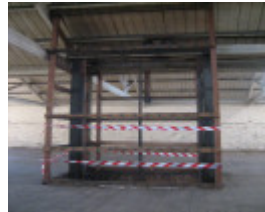
61-9 A'Beckett St lift first floor MZ 24 05 2007
