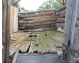
Raised floor and remnant mud and brick pugging to the eastern store
