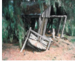
Monmore Vineyard and Buttery Factory, ruined former farm building, pictured 22 July 1994
