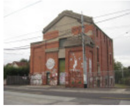
Ascot Vale Substation
