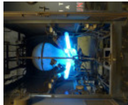
Mercury arc rectifier operating as a number 55 tram approached
