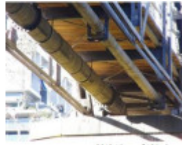
Walmer Street Bridge - pipe from Dights Falls Scheme suspended under bridge - 2019
