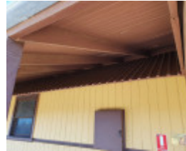
2022, Type A ventilated roof on the Former Irymple Railway Station building showing the batted timber inner roof and ventilator
