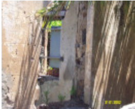
23280 General Store Ruins Byaduk 0401
