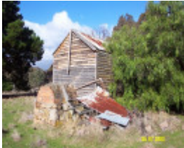
23404 Ruined House Mirranatwa 1138
