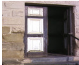
former telegraph office & faulder watson hall barker street castlemaine detail front door telegraph office
