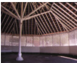
infant building & shelter shed coburg primary school no 484 bell street coburg interior of shelter feb 98
