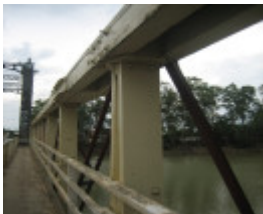
Barham Koondrook Bridge_Koondrook_Feb 2007_mz_Truss Connector Detail
