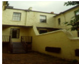
clarendon terrace rear dividing wall sw apr1999
