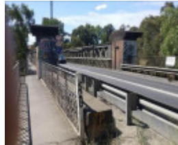
Chandler Highway Bridge looking to the north (City of Yarra) from the southern side of the bridge (City of Boroondara).jpg
