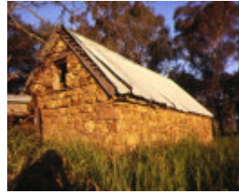
stone cellar at faithfuls creek hume hwy euroa rear view prior to damage
