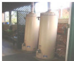
h01204 h1204 166 bellair st kensington rheems boilers nov 2003
