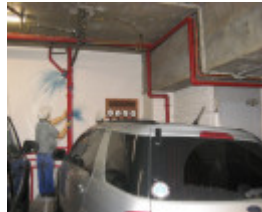
Plumbers & gasfitters garage
