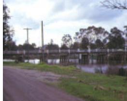
1 bridge broken river benalla side view 1989
