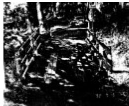
59 - Timber Trestle Bridge Arthurs Creek Eagles Nest Rd - Shire of Eltham Heritage Study 1992
