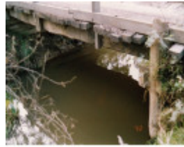
Timber Trestle Bridge Arthurs Creek Eagles Nest Rd Colour 2 - Shire of Eltham Heritage Study 1992
