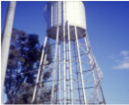
h01833 water tower and tank millard street wangaratta tower and pipeworks she project 2003
