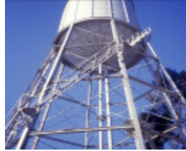
h01833 water tower and tank millard street wangaratta close up she project 2003
