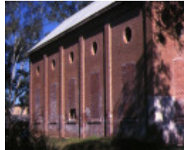
billabong pumping station nichols point irymple mildura side view jun1982
