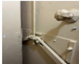
2023. Bank vault locking mechanism to ground floor.
