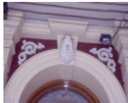
h00116 old colonists hall lydiard street north ballarat death mask over front entrance she project 2004
