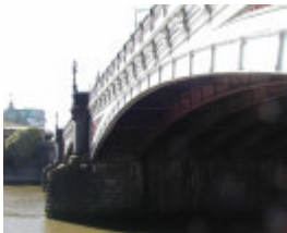
h01447 princes bridge st kilda road over yarra river melbourne below she project 2004
